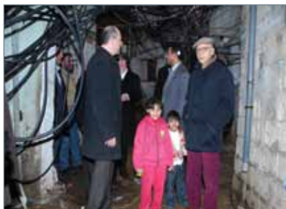
Dangerous electrical wiring is everywhere in Bourj al-Barajneh
